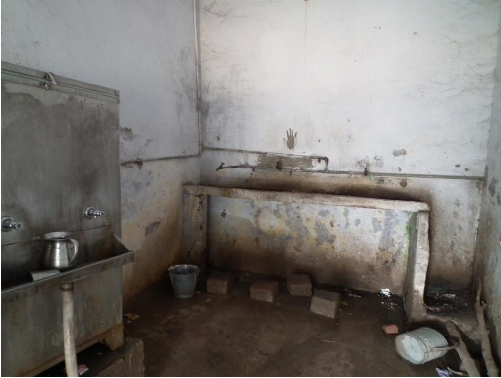
Drinking Water Arrangement at Govt. School Bhakhar Pur
