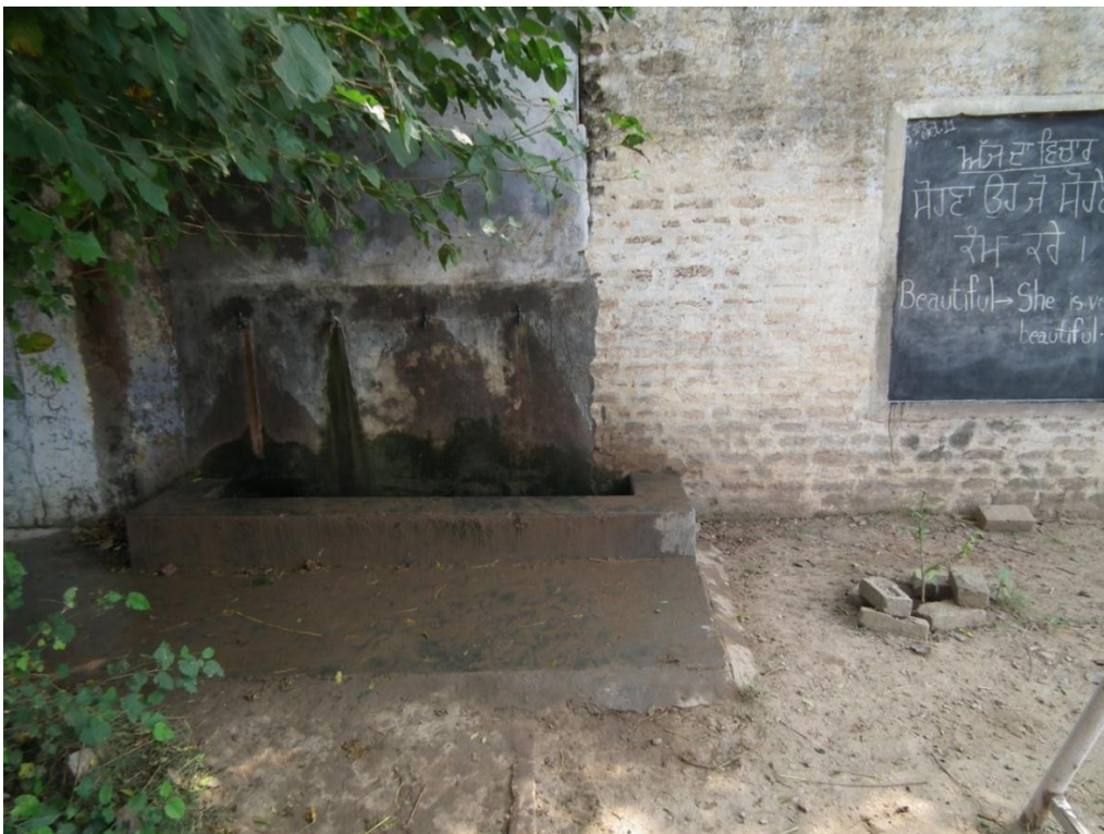
UNHYGIEIC ( WATER ARRANGEMENT ) GOVT. ELEMENTARY SCHOOL, RURKI PUKHTA
